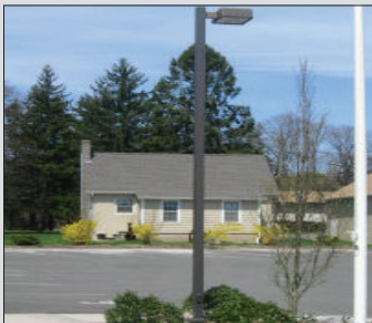
parking lighting on Boston Post Road East
