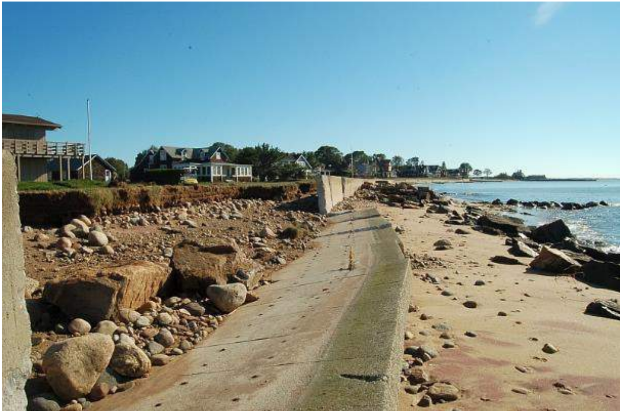
Figure 7: Collapsed seawall in Fenwick caused by Tropical Storm Irene
