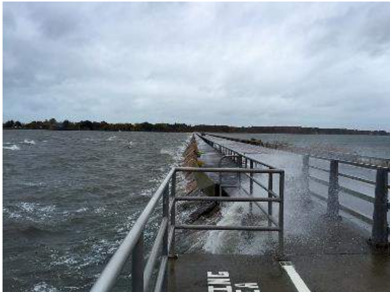
Figure 24: The Causeway, an important arterial State road, is at risk of flooding during coastal storms
