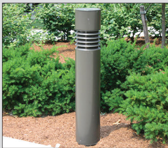
pathway lighting at the Town Hall
