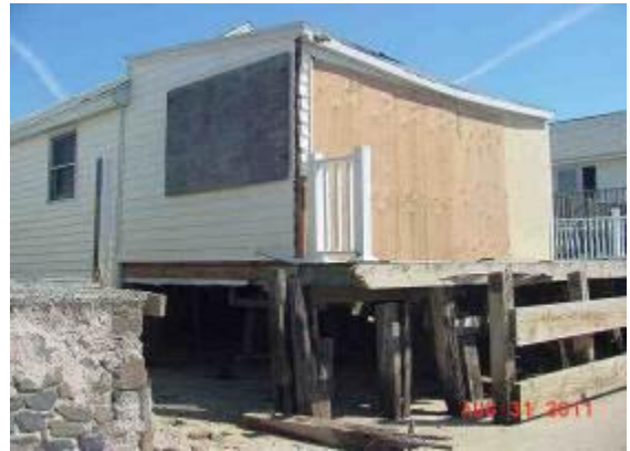
Figure 9: 2011 Tropical Storm Irene damage - Damaged house on Beach Road.
