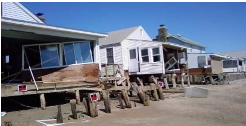
Figure 10: Coastal Storm Damage Examples of damage at Chalker Beach caused by Tropical Storm Irene, September, 2011.
