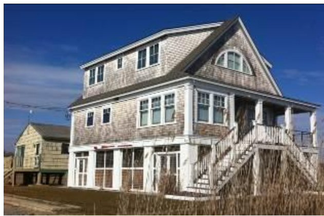
Existing homes. Mitigation of older homes vulnerable to coastal flooding and storm surge includes elevation of existing structures. This view shows one house recently elevated with another in the background, which needs to be elevated.
