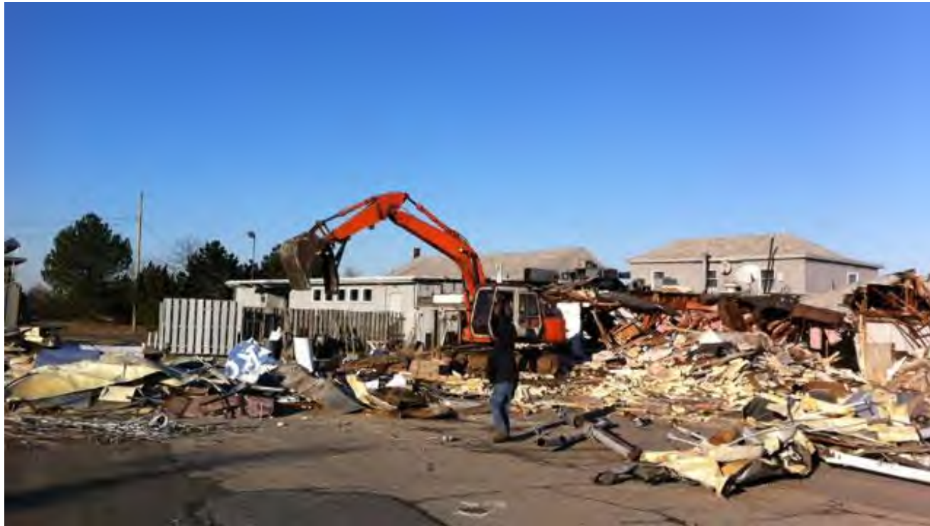
Demolition of Dock and Dine on Saybrook Point after Sandy image from http://www.wfsb.com/story/24398944/demolition-begins-at-dock-dine-in-old-saybrook
