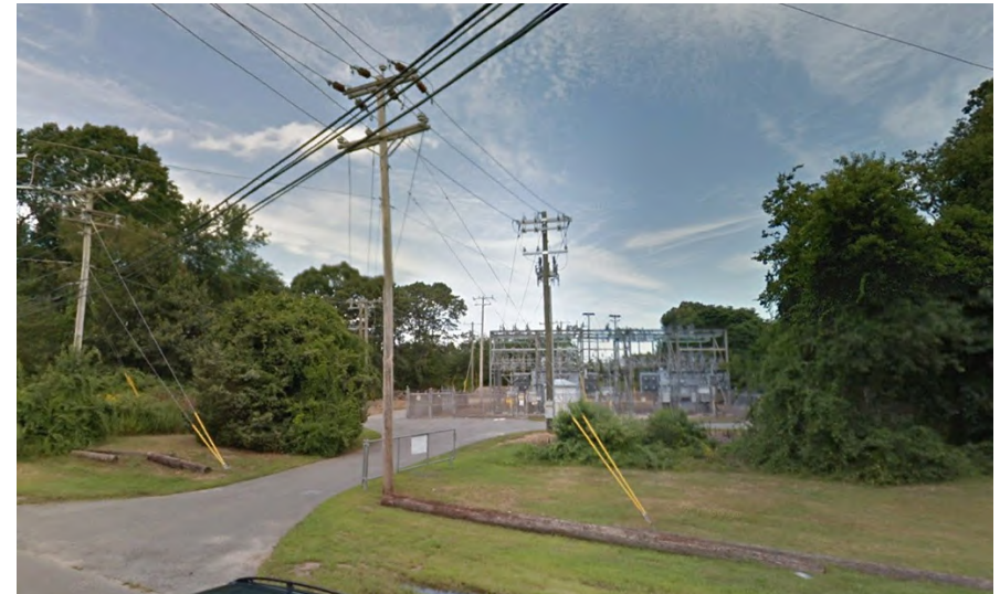
Figure 3-6: Vicinity of Eversource Elm Street Substation; Ground Surface Elevation +/- 14 feet NAVD88 (top image)
